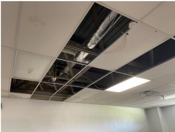
Damaged tile in classroom where maintenance personnel are tracking gutter and downspout failure.
