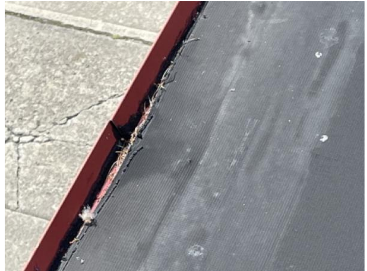
Frayed edge of EPDM at roof's edge where water is running down into building.
