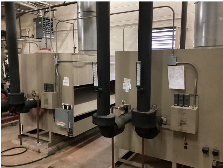
Outdated boilers that serve the building. Only one is currently operational.
