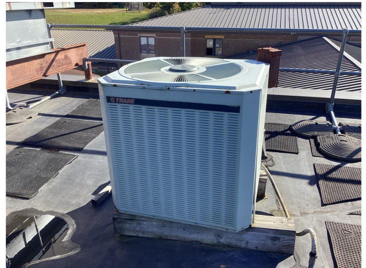
Split system HVAC unit to be replaced.
