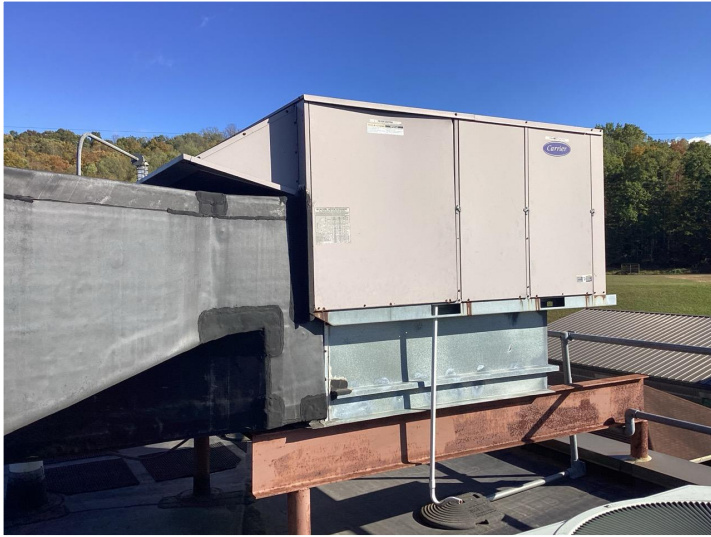
Rooftop HVAC unit that serves the gymnasium in need of replacement.
