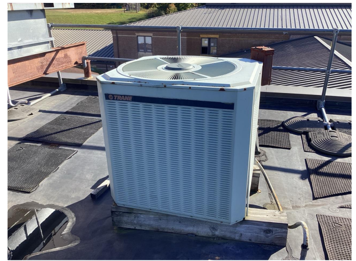
Split system HVAC unit to be replaced.
