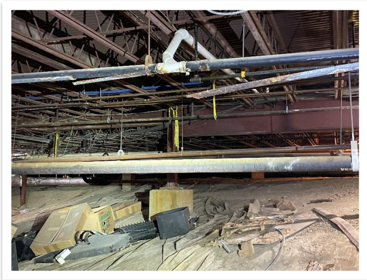
The plumbing is located in a crawl space under the facility with some existing pipes underground and hard to find.
