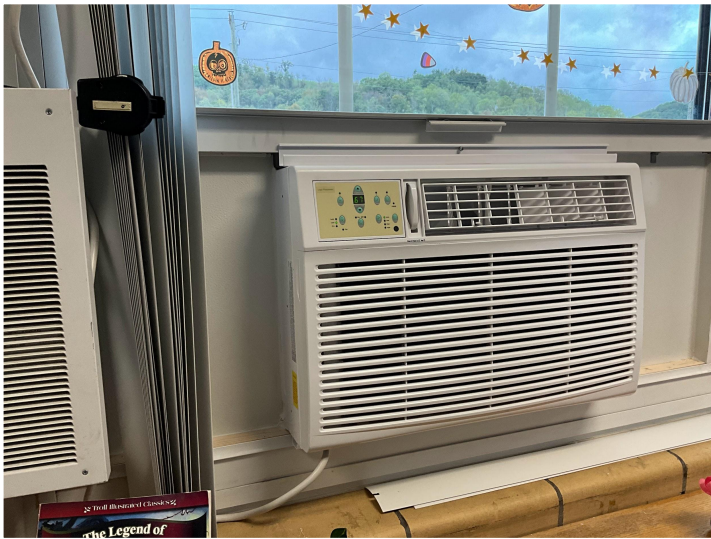
Window AC units supplement the current HVAC system. These AC units will be switched out to heaters during the winter.
