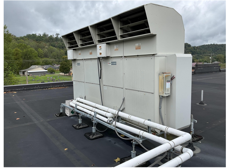
The current HVAC is susceptible to frequent power outages, which damage the compressors and controls.
