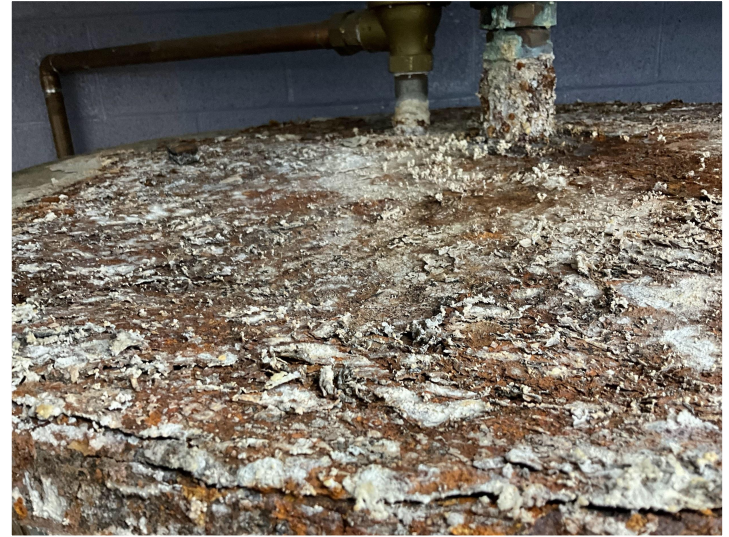
The top of the water tank is completely rusted/corroded.
