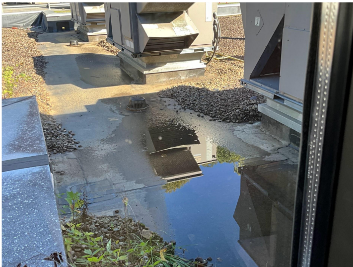
The EPDM roof is ~28 years old and has been leaking into classrooms, hallways and the science lab.
