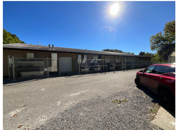
The metal roof (1988), which covers the clinic and new animal processing center, has been leaking since 2015.
