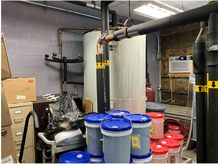
The 500-gallon water tank, which serves the main building, is ~25 years old. Leaks have developed from the tank and lines.
