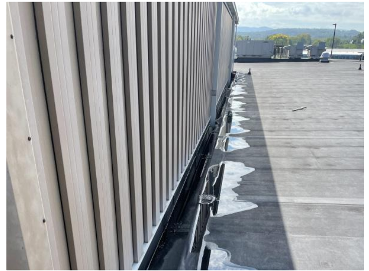
Water pools at roof trench. Weathering stresses seams and water penetrates walls below.
