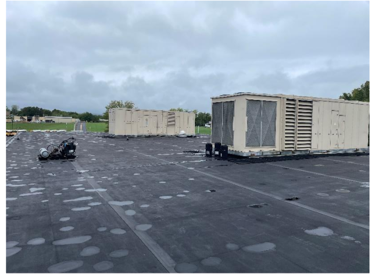
Mammoth roof top unit showing ongoing replacement of compressors. Replacement parts are becoming obsolete.
