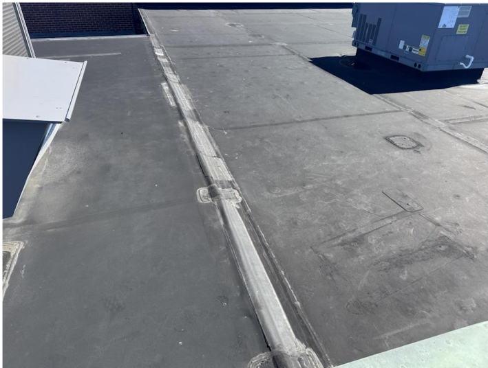
Seams are failing since they do not have sufficient overlay.
