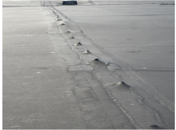
Fasteners are punching through roof from underneath.
