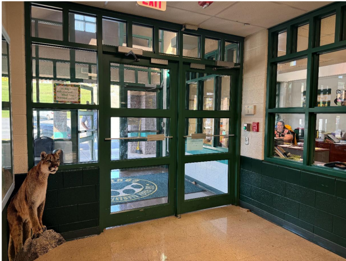
At East Hardy ES, the scope is to replace hardware, repair doors and windows and repaint all framing.
