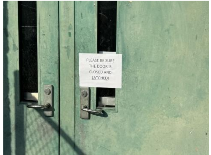
At East Hardy ES, hardware is malfunctioning, and doors often do not fully close.
