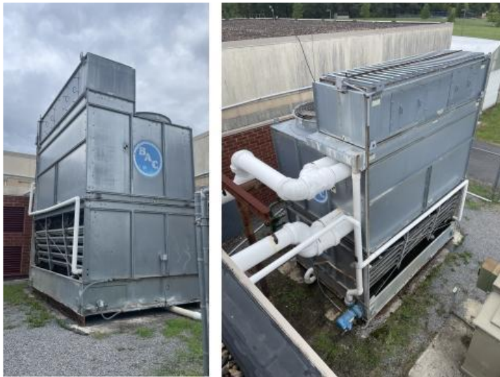
Open Loop Cooling Tower where water runs over fill to cool, and it is collected in the basin below.
