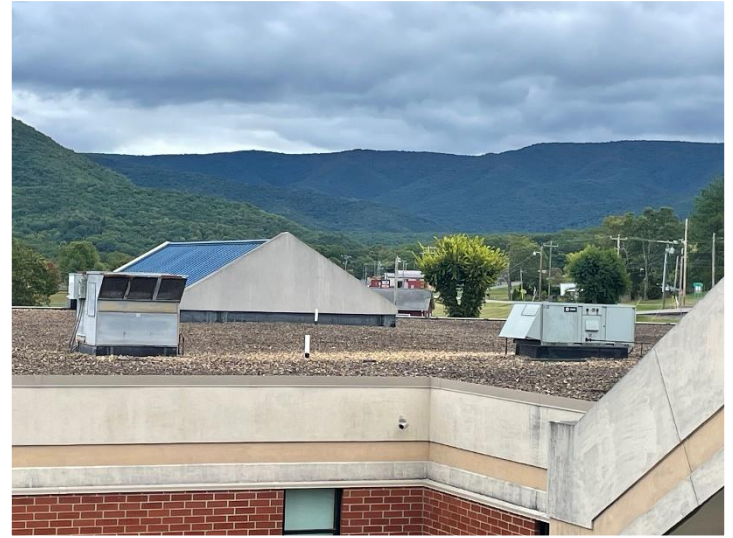
The roof to be replaced with MIP funds and some equipment that will be affected.
