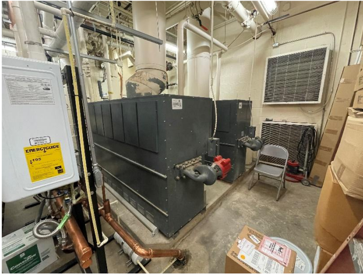
Two boilers to be replaced at school.
