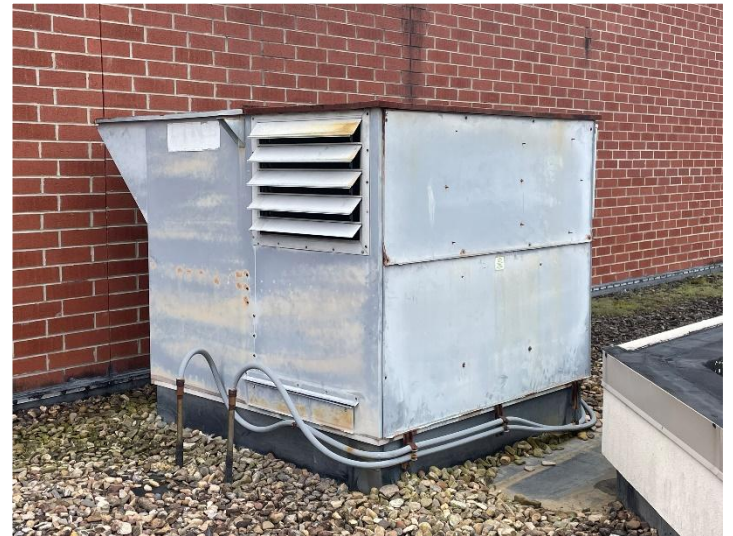
One of the three Dedicated Outside Air System (DOAS) to be replaced.
