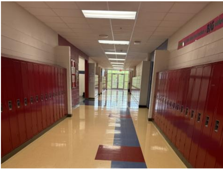
At Mountaineer MS, a wing of the facility will be renovated for PreK/ K with restroom in classrooms
