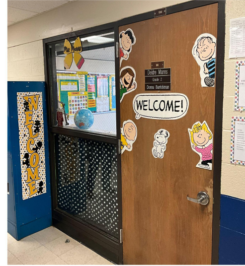
Classroom entrance sidelights are a safety concern, as they allow unhindered visibility to the entire room.
