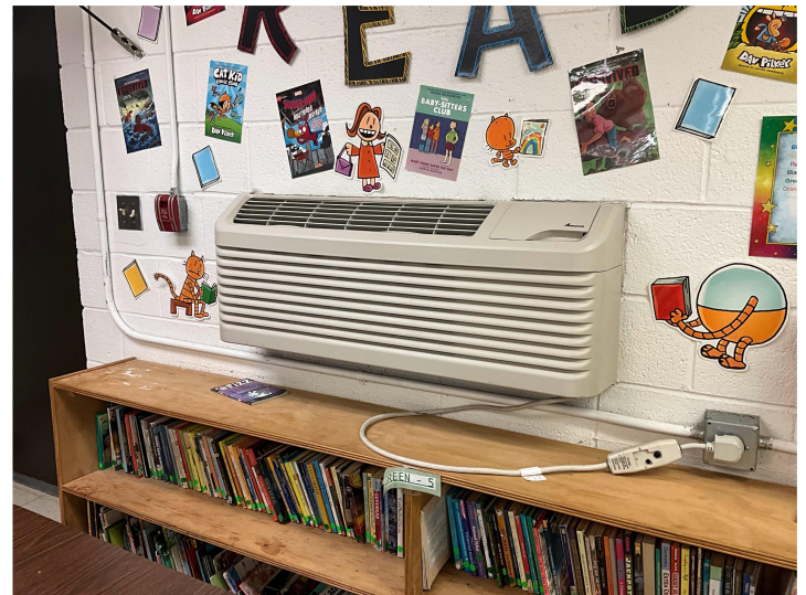
All classrooms have PTAC units which do not meet current WVDE indoor air quality requirements.
