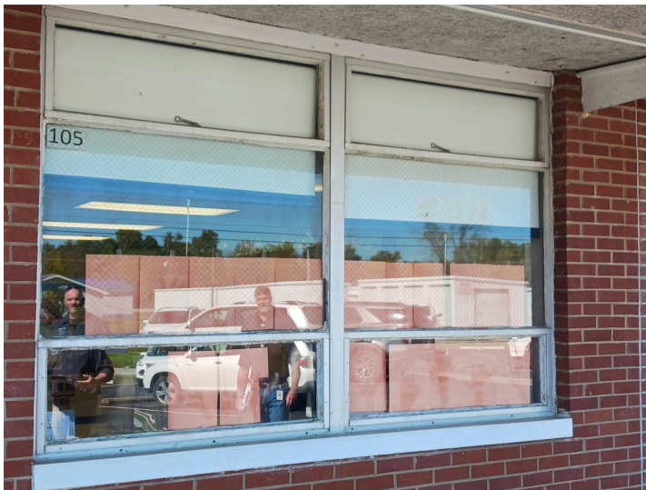
Exterior windows are original to the school being built in 1960 and are not energy efficient.
