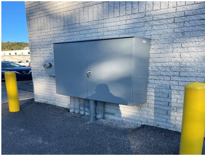
Jackson county has already spent $3.6 million renovating the HVAC and electrical system at this facility.
