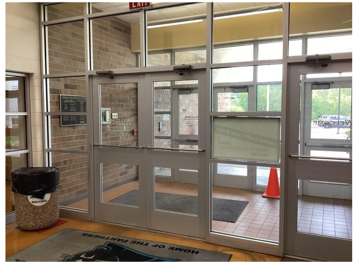
Interior view of existing main entrance to be renovated into a safe school entrance.
