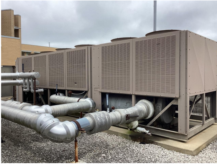
Existing chiller, original to the facility, at the end of its operational lifespan.
