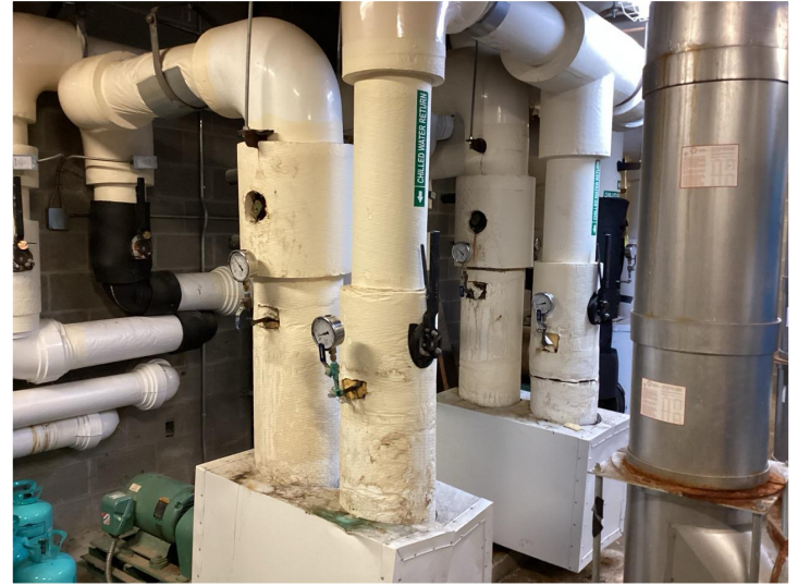
Upgrades to plumbing and electrical components to accommodate the new chiller will also take place.
