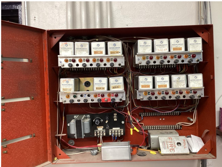
Outdated fire alarm panel which cannot support any new devices or communicate with modern systems.
