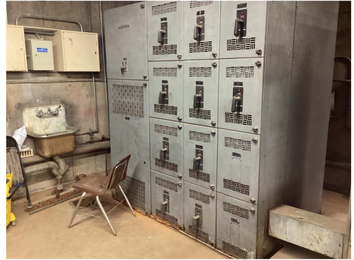
Electrical Main Distribution Panel (MDP) which is original to the building and far beyond its intended life.
