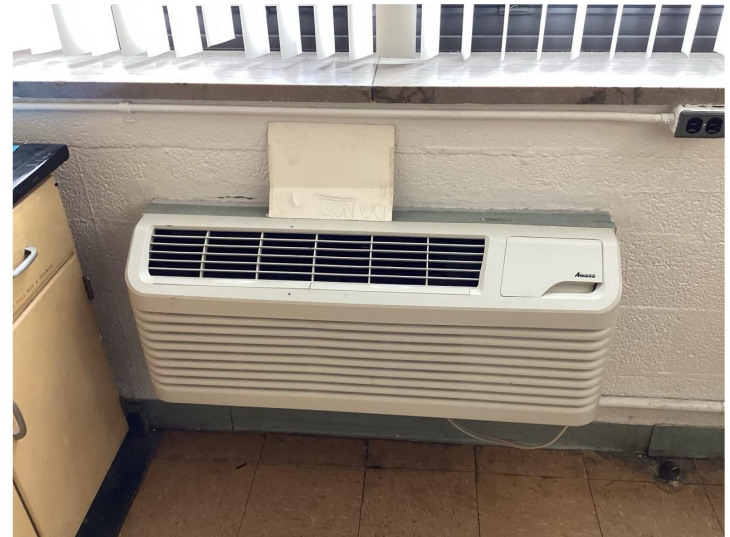
The existing HVAC system and controls are beyond their operational life expectancy.
