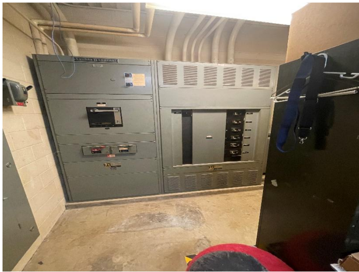
The HVAC, electrical upgrades and flooding on the exterior of school keep kids out of school.
