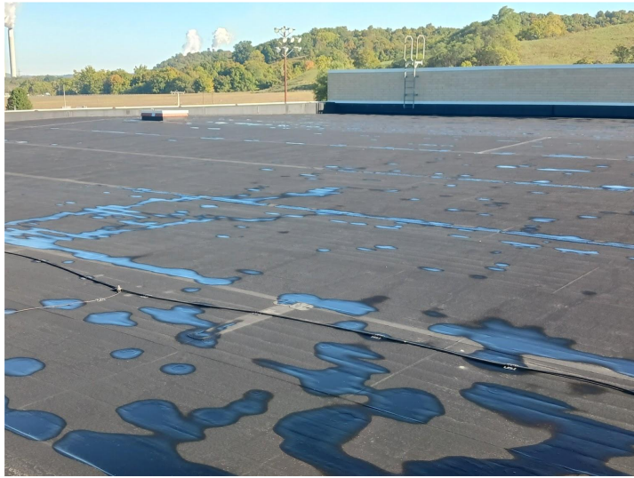
Water has been leaking into the school, with some classes having to be displaced.
