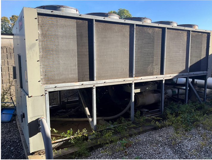
The Intermediate School's mechanical chiller has surpassed its optimal 20-year lifespan. The unit was installed in 2003.
