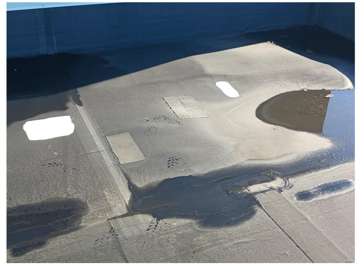
The existing roof showing patches and separation of the membrane from the insulation/deck.
