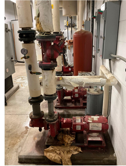
Additional mechanical equipment is at its end-of-life cycle according to ASHRAE Life Expectancy Charts.
