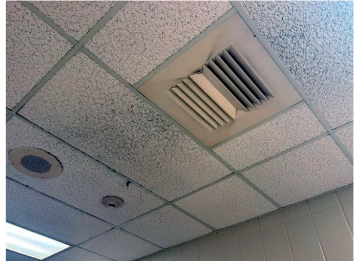
The lack of ductwork for return air creates more dust/dirt particulates, since air gets pulled into ceiling cavity.
