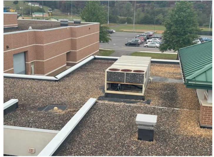
The rooftop unit serving the main office and entry area will be replaced.
