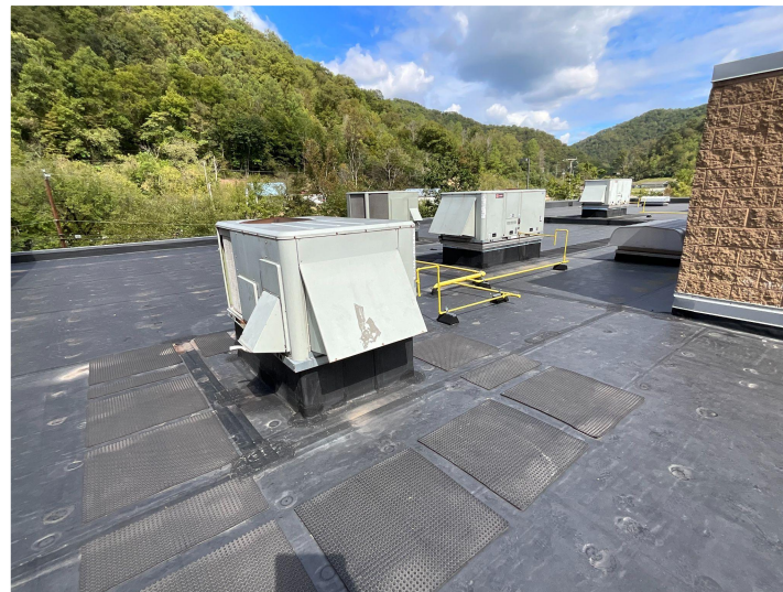
Rooftop units, of differing brands, are at the end of their life-expectancy, and are not operating properly.
