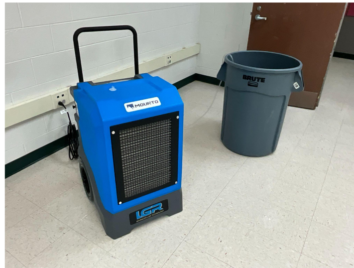
The county has resorted to renting industrial dehumidifiers, each filling a 32 gallon container per day.
