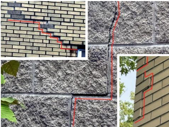
There has been repointing of mortar in the past, but cracks are reappearing that travel through bricks and block.
