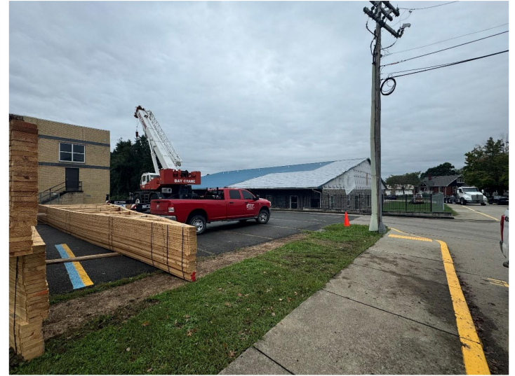
The 6 th grade annex building had a roof and truss replacement this summer/ fall due to water issues.
