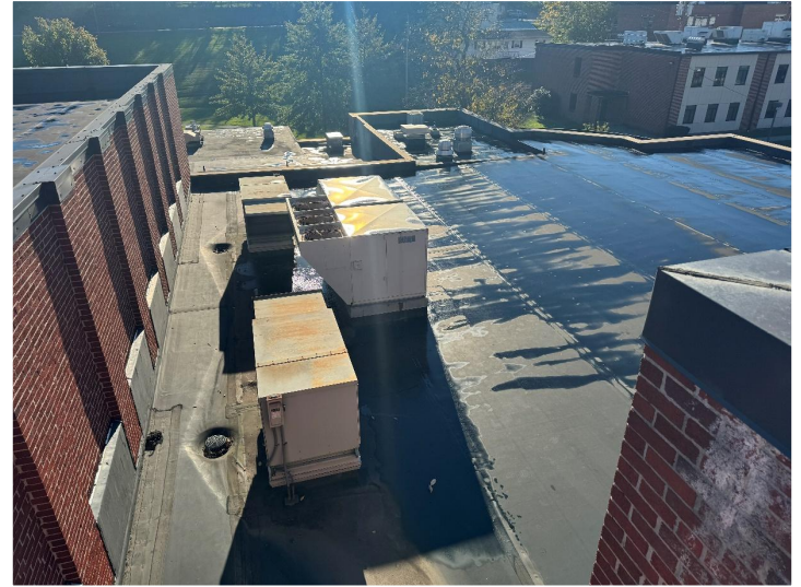
The roof overview that is proposed to be replaced at Berkeley Springs HS.
