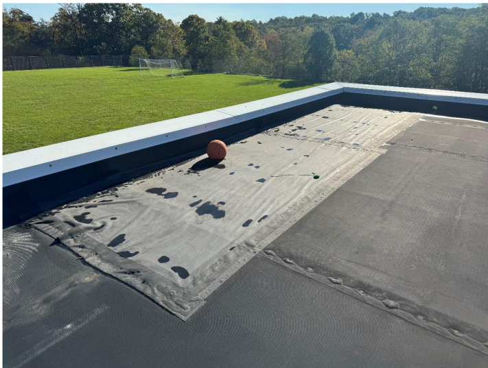
At Warm Springs Intermediate, large patched area have seams still failing.
