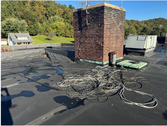
Areas where EPDM is failing at flashing, HVAC curbs, and parapet at Berkeley Springs HS.
