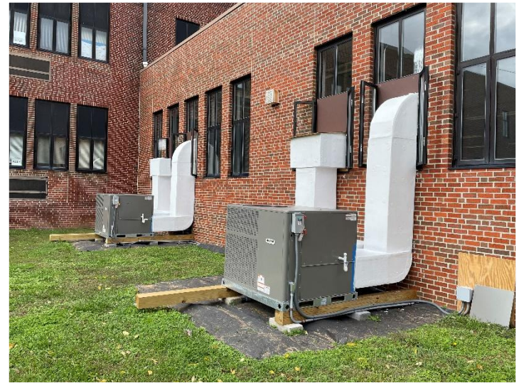
Temporary equipment for air conditioning in the cafeteria of Berkeley Springs High School.
