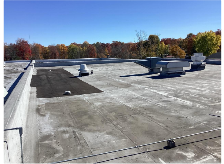
The existing roof has been patched and sealed several times over the years and needs replaced.
