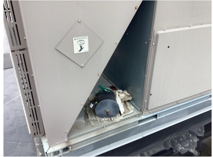
This RTU had recently been serviced, with a defective part set aside for troubleshooting / replacement.
