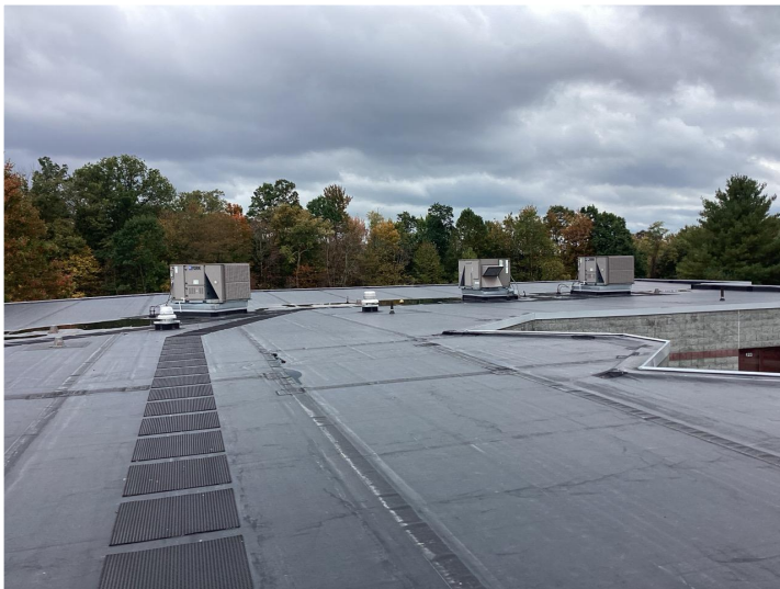
All of the RTUs were replaced over 10 years ago, but the equipment is reaching the end of its useful life.
