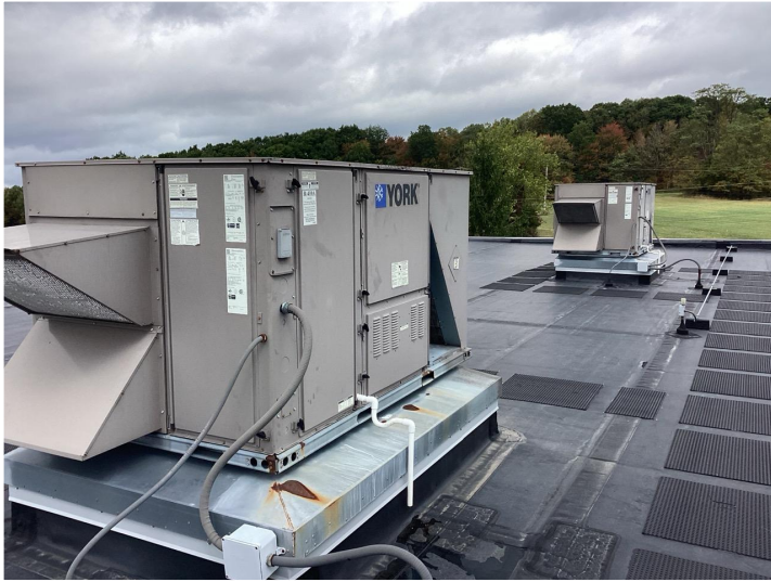
The rooftop units (RTUs) at Panther Creek Elementary School have begun to show signs of aging and deterioration.
