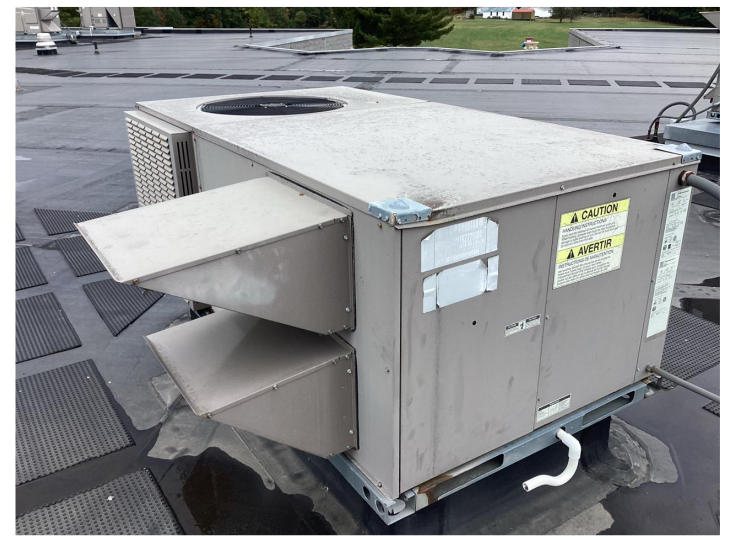
The coolant that these units require has become outdated, and the HVAC building controls have become obsolete.
