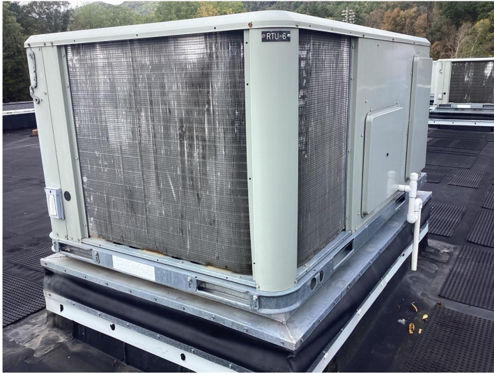
Aging rooftop units (RTU) at Brandywine Elementary, situated upon an EPDM roofing membrane in need of replacement.
