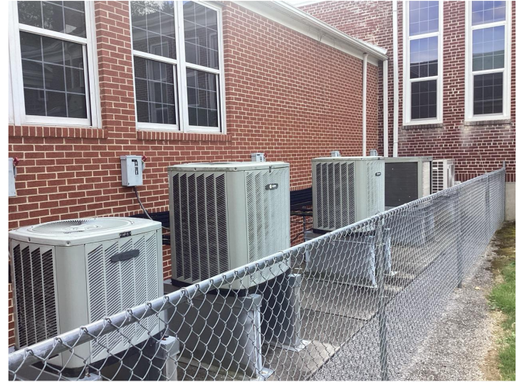
Mini-split system HVAC units at Brandywine ES that are approaching the end of their useful life.
