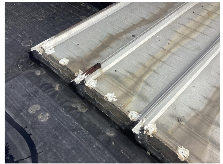
The worst areas of water infiltration in the building are located where the metal roofing transitions to other roofing sections. These areas would also be addressed.
