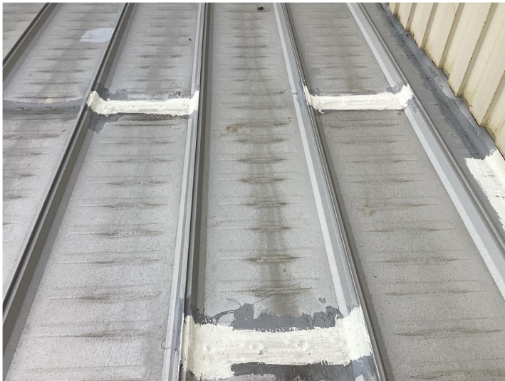
The metal roofing over Pendleton County Middle/High School has been patched in numerous places, with leaks throughout the building.
