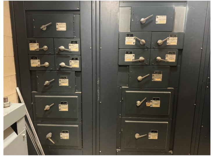
Phase III of the electrical renovation involve the replacement of the switchgear in the school.
