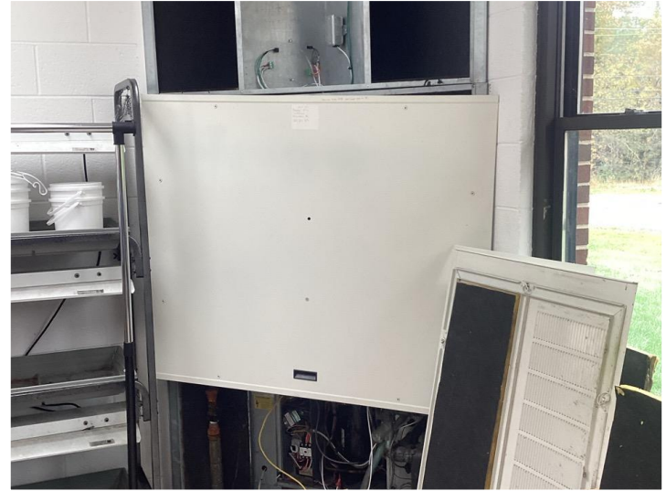
A water source heat pump that has been taken apart for repairs. Replacement parts had not yet been found.
