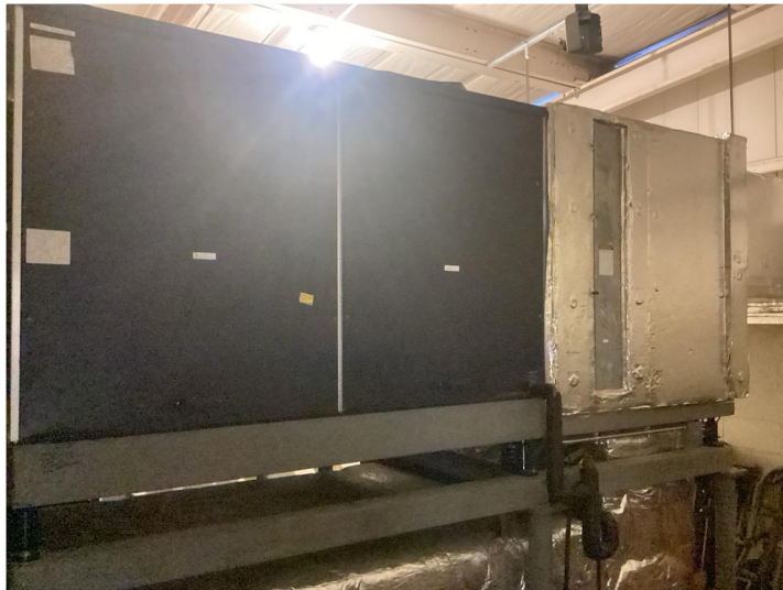
One of two large HVAC units that condition the gymnasium.
