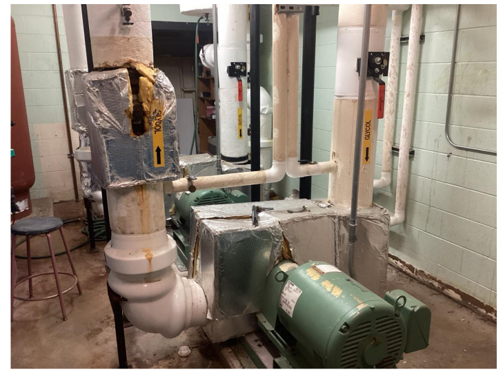
Aging pump assembly that transmits the glycol solution throughout the building to maintain the geothermal system.
