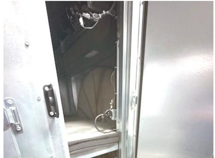
Recovery wheel in unit that was working at the time of SBA staff's visit.
