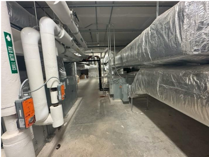
Large ducts to air handler unit.
