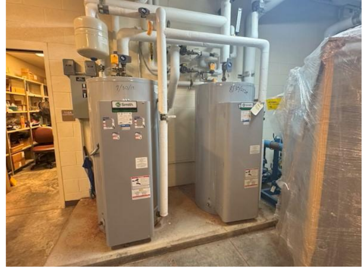
Existing electric boilers.
