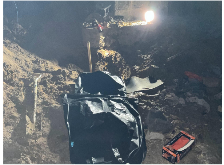
The sewage lines (original terra cotta) constantly back up, with odors infiltrating the school.
