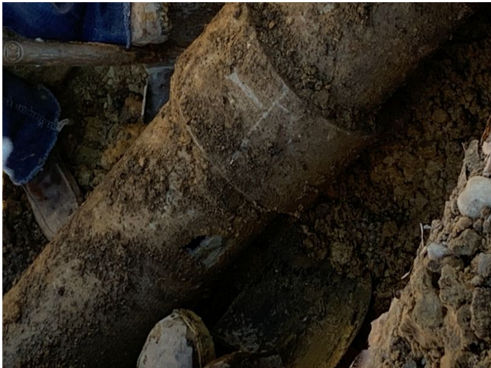
This photo was taken during the most recent water line break at the school.
