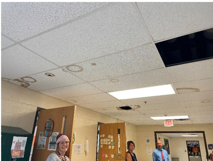
The corridor where leaks continue to occur.
