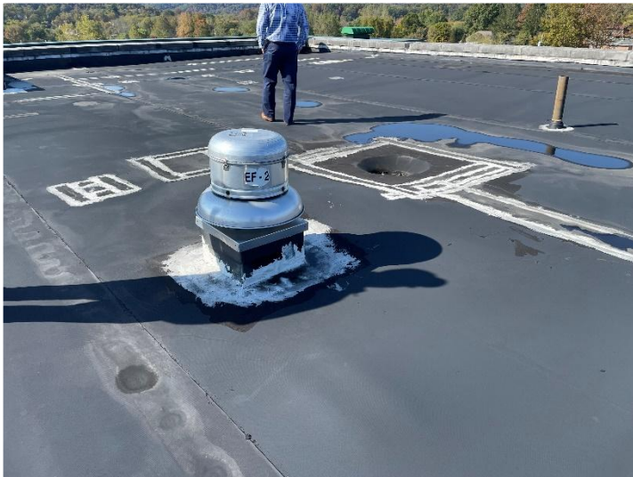
The roof where seams have been patched and reglued.
