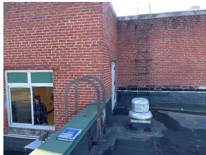
Current access to the roof is on a chair then out a window. Access door to be operational and new ladders on roof.
