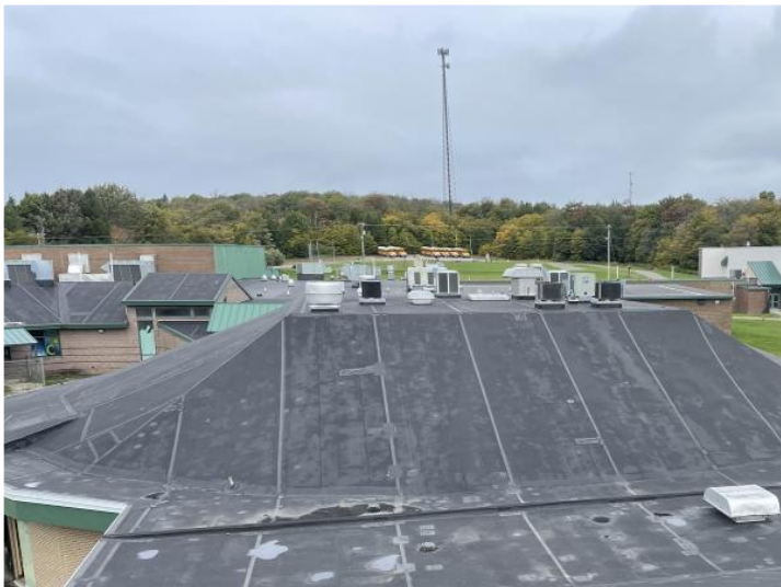
HVAC equipment over vocational center to be replaced.
