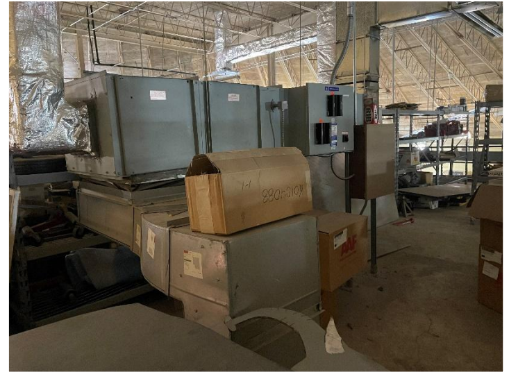
View of equipment and ductwork above classroom under the roof.
