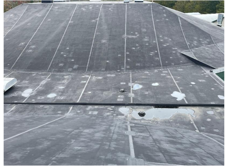
Multiple patches are all over the vocational roof.
