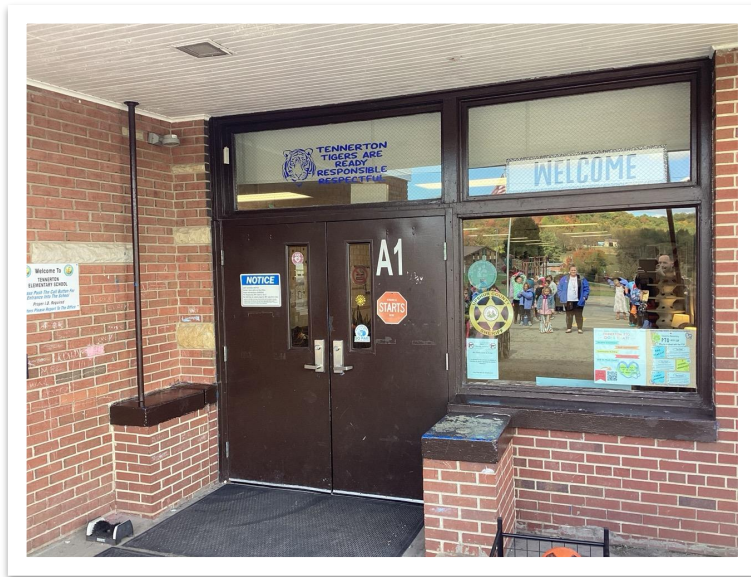
Existing main entrance to the facility to be renovated into a safe school entrance.
