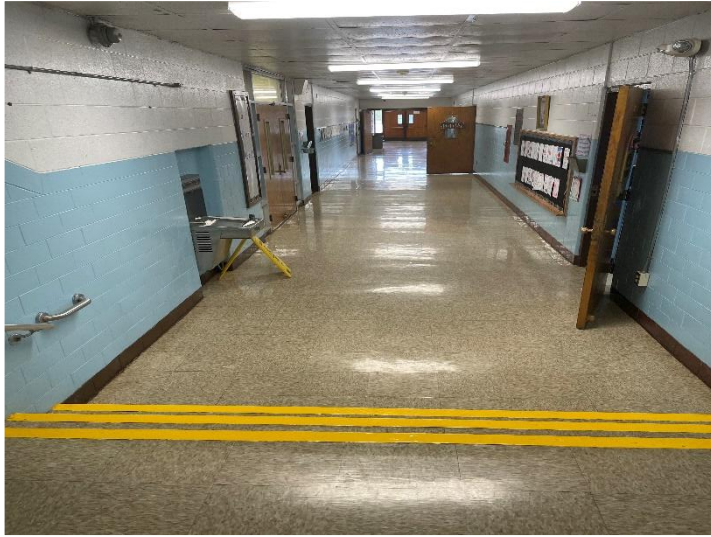
The existing school has many ADA issues throughout the facility.
