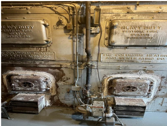
Existing coal burning furnace that was converted to gas in the past few years.
