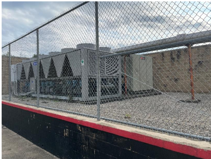
The county has replaced one chiller with local funds. The other chiller has continuous issues and needs to be replaced.
