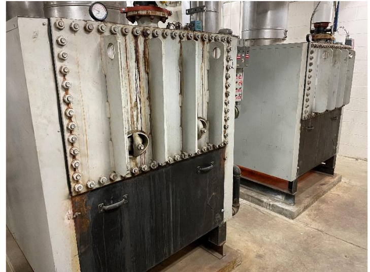
Boilers are original and has exceeded its life expectancy..
