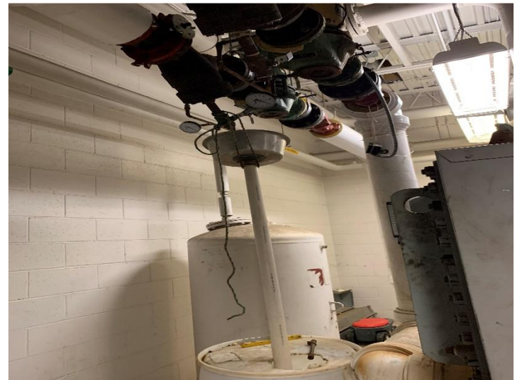
This will help the facility to improve air quality and will help maintenance to work on preventative issues.
