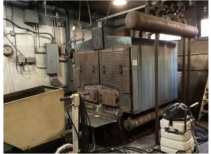
Coal-fired furnace used to heat Ansted until last year, when its use was discontinued.
