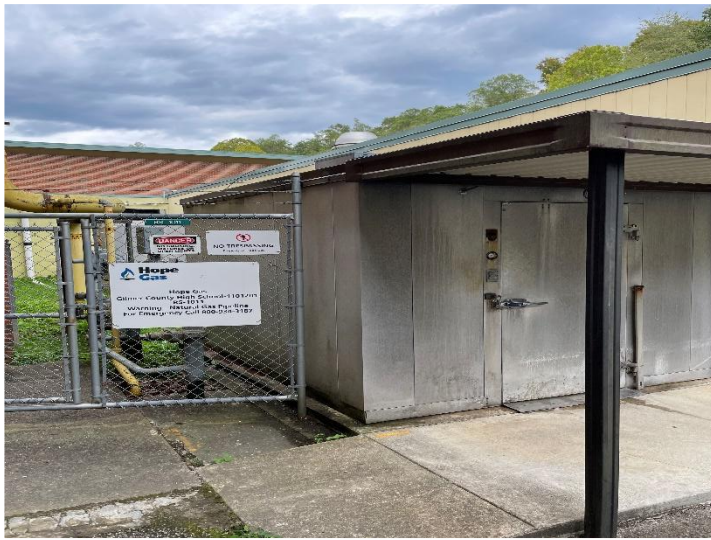
The cooks have to go outside to access the refrigerator and dry storage area.
