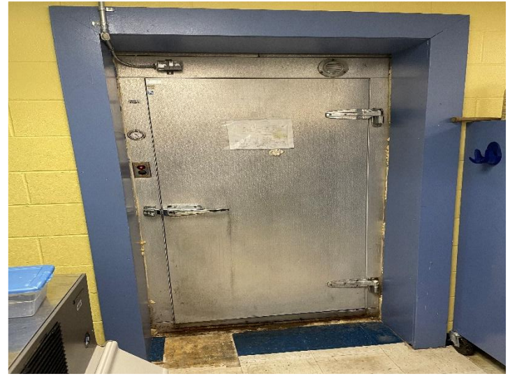
The freezer door get stuck because the concrete slab is failing outside.
