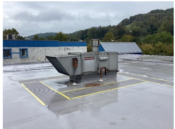
Most of the units are showing considerable signs of rust and deterioration.
