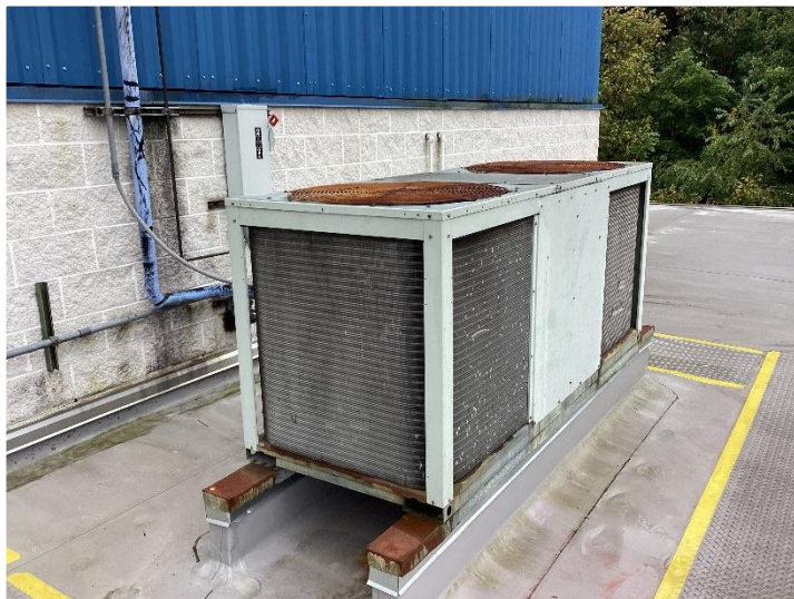
This unit was not running at the time of visit. Several units have failed at the school.
