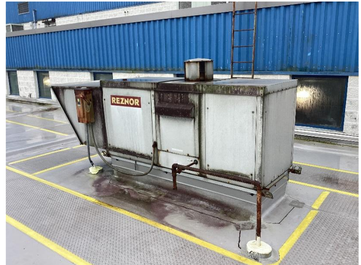
Example of aging rooftop unit (RTU)
