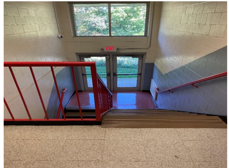
An elevator will be added in the two-story wing for ADA compliant..
