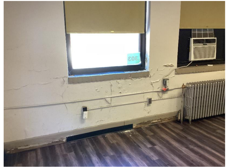
Walls, ceilings, and floors are showing major signs of deterioration due to age and water infiltration.
