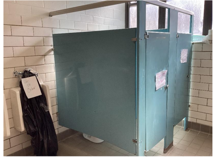
Out of order restroom due to plumbing issues.
